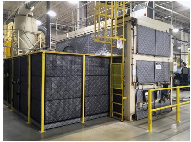
Sample Noise Engineering Controls
